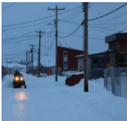
Power-pole distribution in a community
