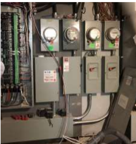
Splitter-feeding multiple disconnects for individual houses
