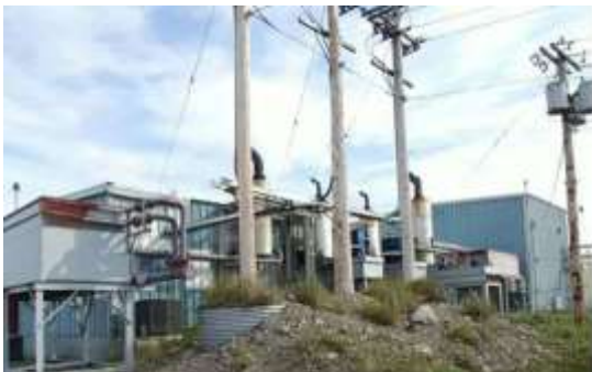
Transformer and Distribution: Overhead power poles
