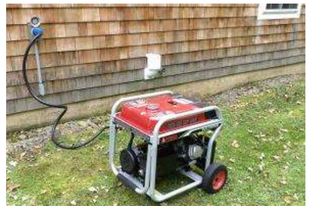
A mobile generator connected to a house
