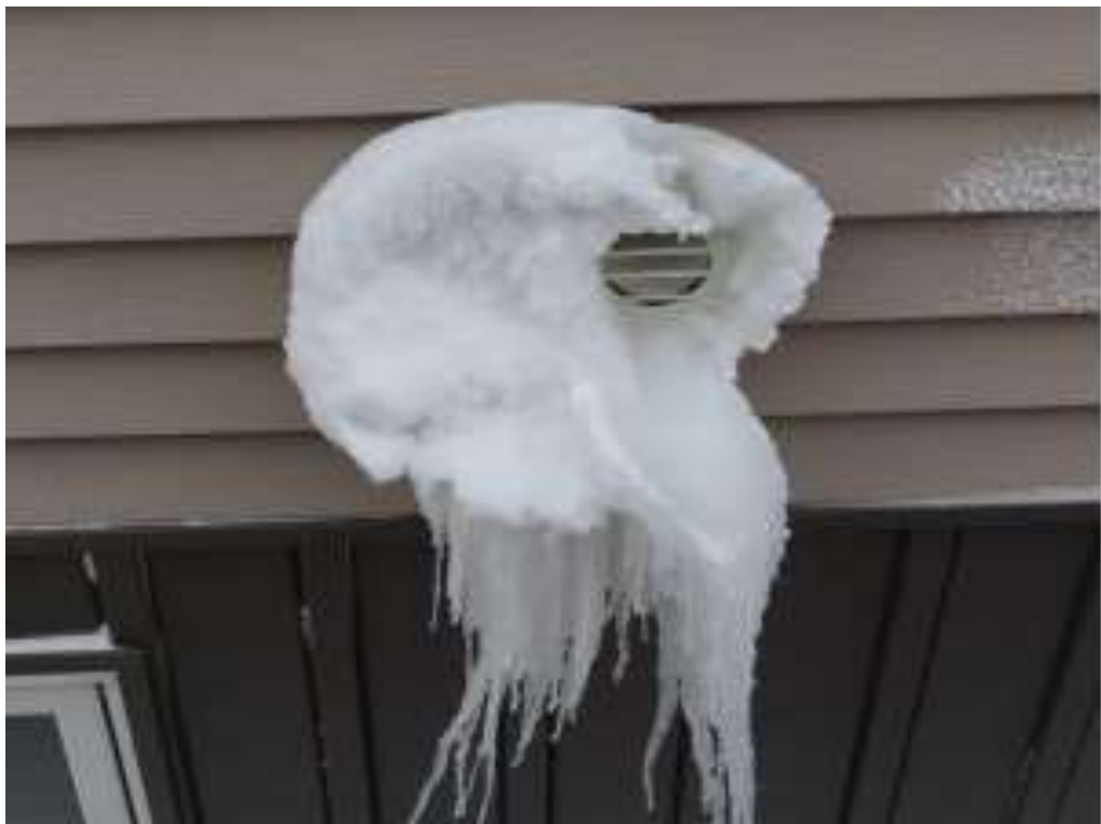
The exhaust and air intake for this furnace was frozen over
