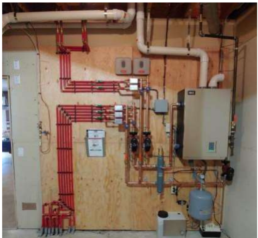
Hydronic boiler equipment with pipe manifold
