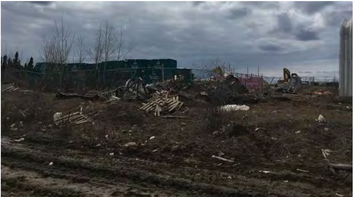
Figure 94 : Construction materials stored outside without protection.
