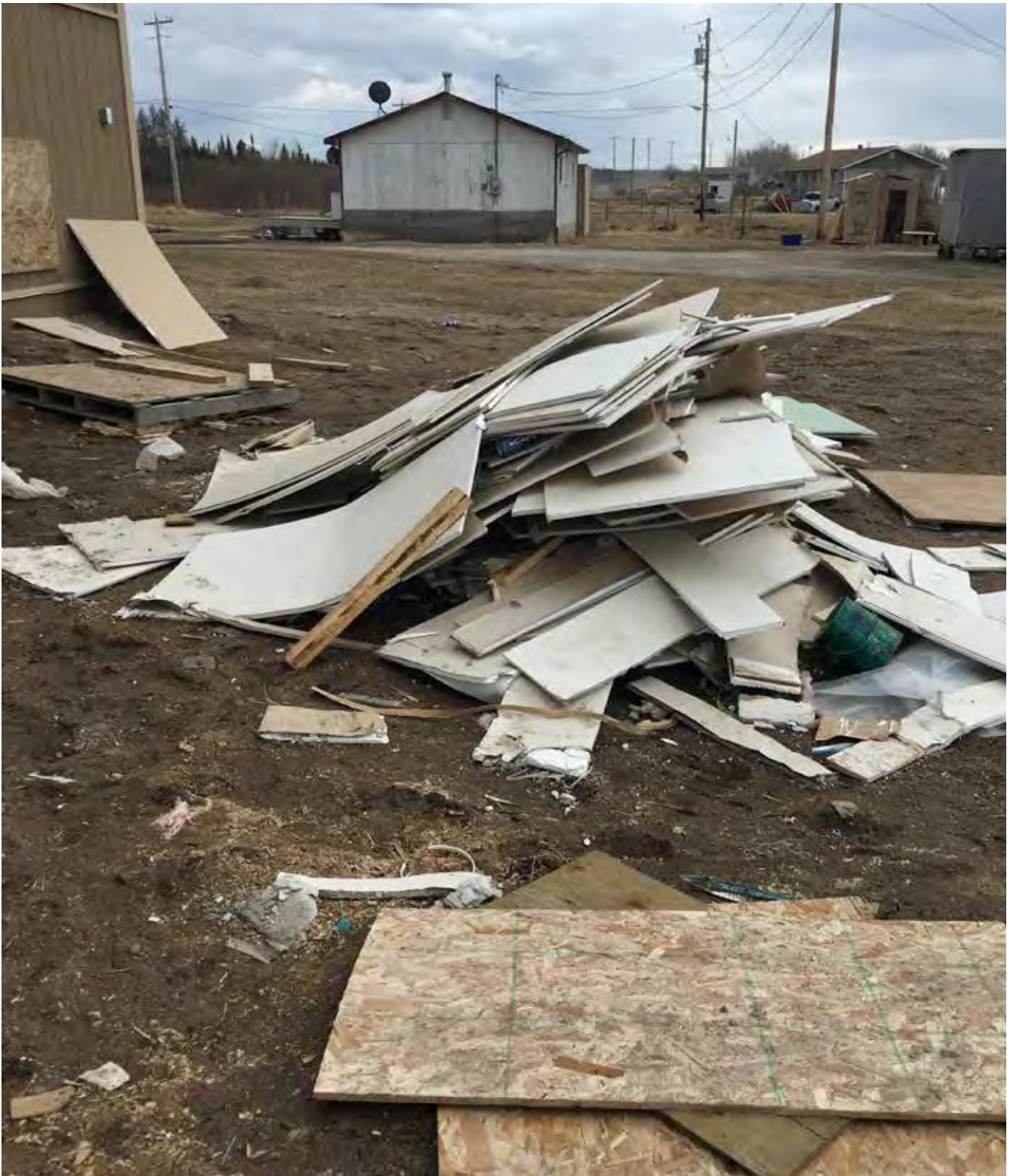
Figure 93 : drywall waste at construction site of new bi-level house.
