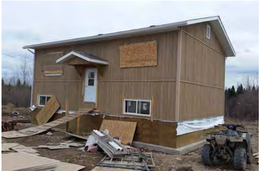
Figure 62 : split-level with broken windows and add-on water tank room
