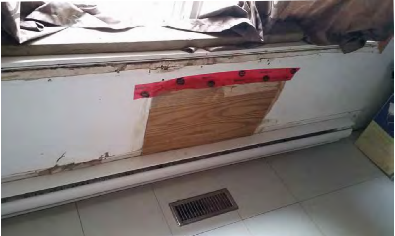
Figure 86 : drywall damage below an improperly installed window
