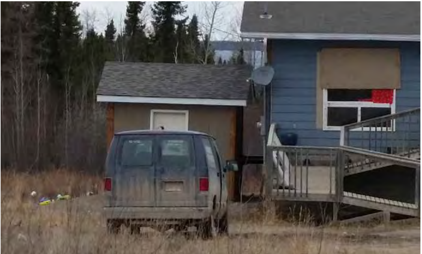
Figure 56 : bungalow with separate water tank shed, the structure should share a wall with the house to prevent freezing pipes.
